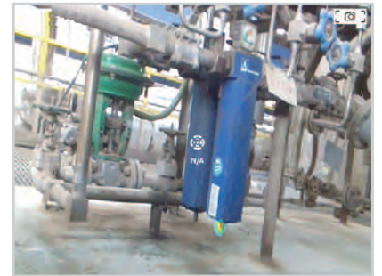
Dry Running gas seals/Nitrogen leak
