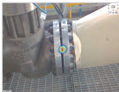
Flange/process gas leak
