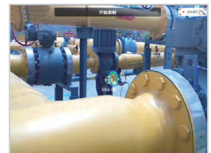
Natural gas valve leak
