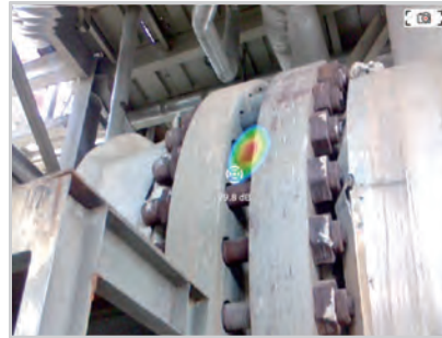
Giant steam flange leak
