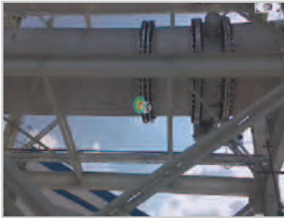
Overhead pipe flange leak
