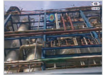
Workshop top pipe joint leak
